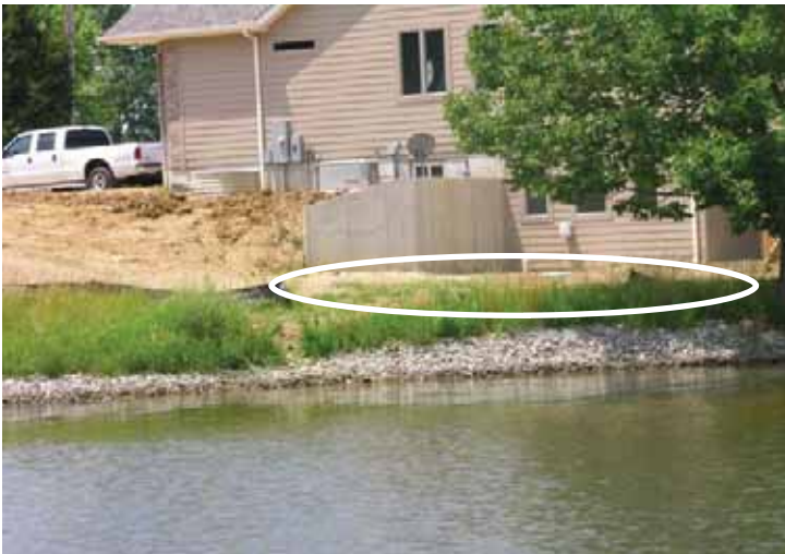
Photograph 9. Lot 759, in Sioux Cove's watershed, had a gap in its silt fence (circled in the photo).
