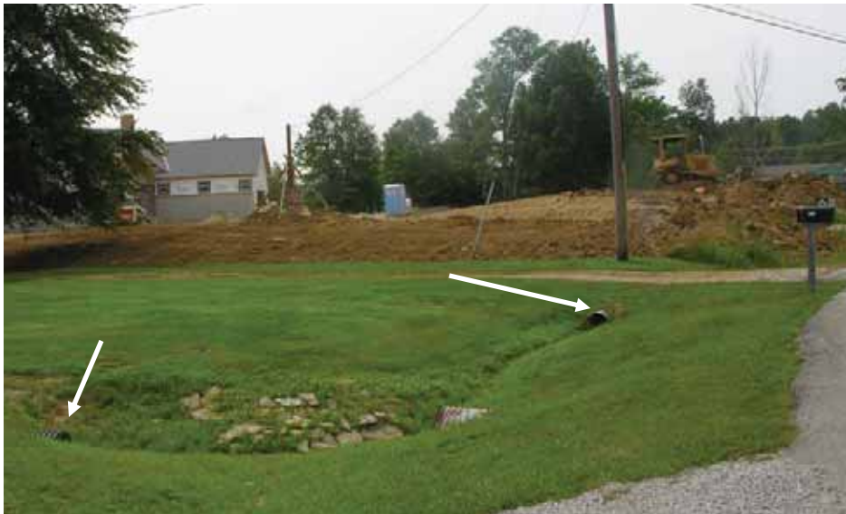
Photographs 31-33. Lot 421 on Cove 11, does not have silt fence in the front or on the sides, where sediment can reach the lake via culverts, indicated by white arrows. Silt fence is present in the rear, but had a gap during our July visit (indicated by circle on lower left photo).
